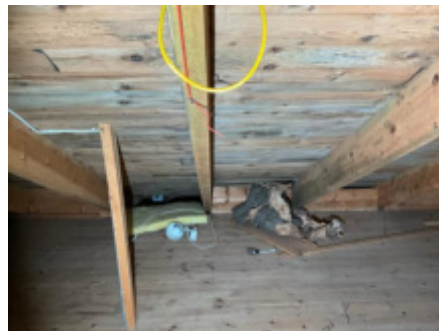
Misfarging i undertaket.
